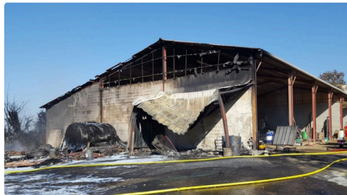
pompier gaz oil 3.JPG
