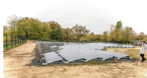
Le champ photovoltaïque
